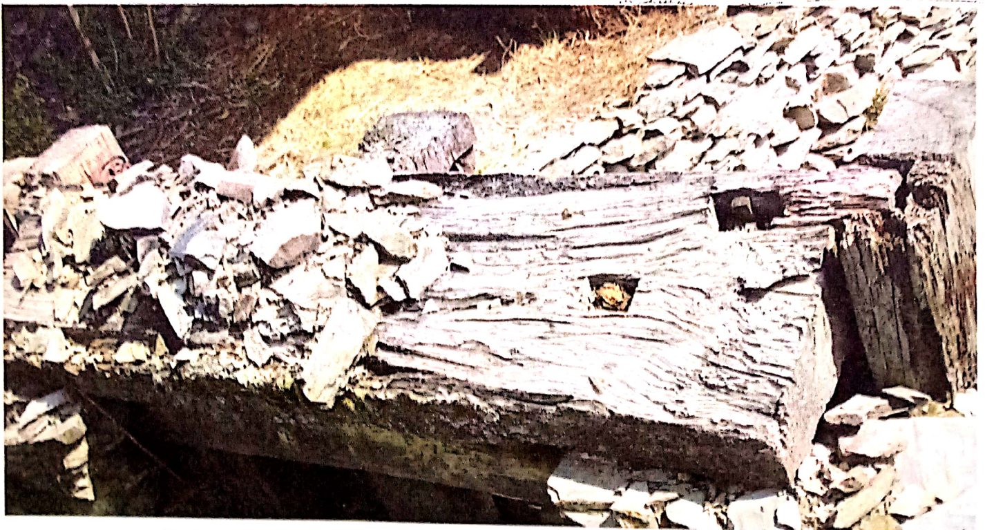
Fig.11: Housed and nailed joints used for fixing the wooden components of Koti Banal architecture.
