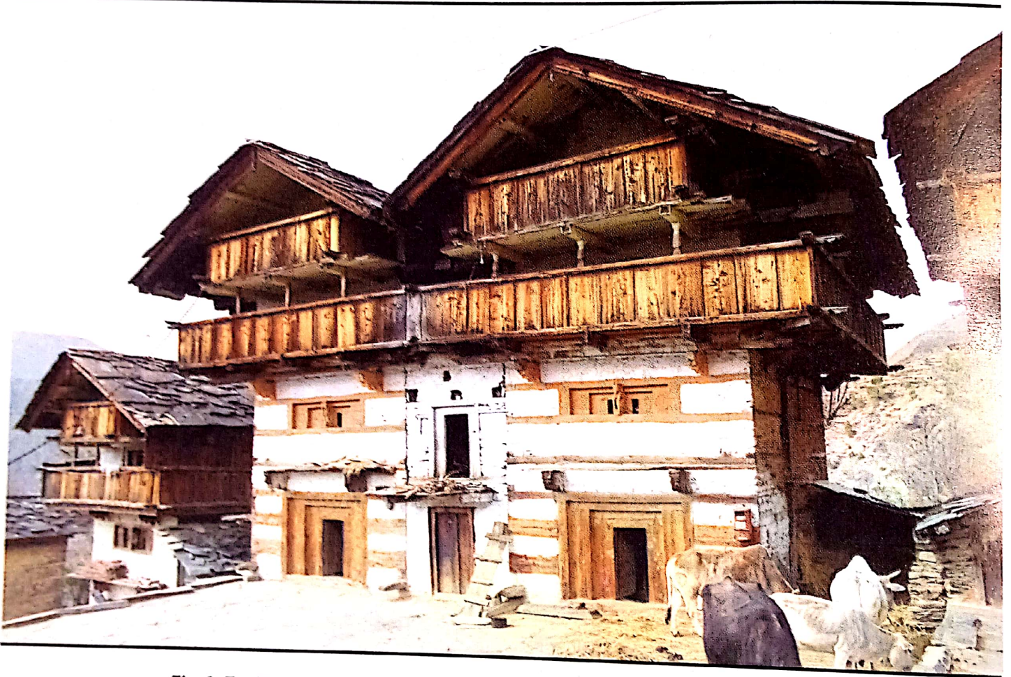
Fig. 6: Tradition in shambles : view of the abandoned multistoried structure at Koti Banal
