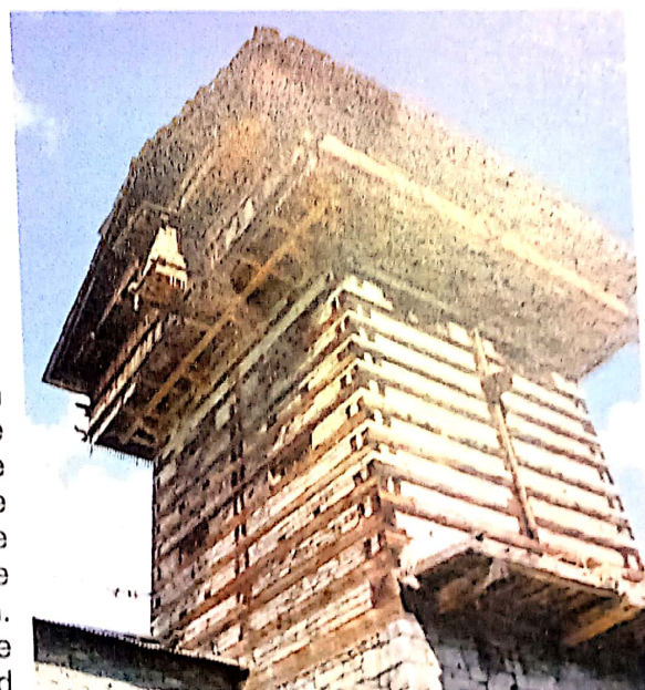
Fig.10: The vertical wooden beam on the side walls is considered to be a seismic safety related provision.
