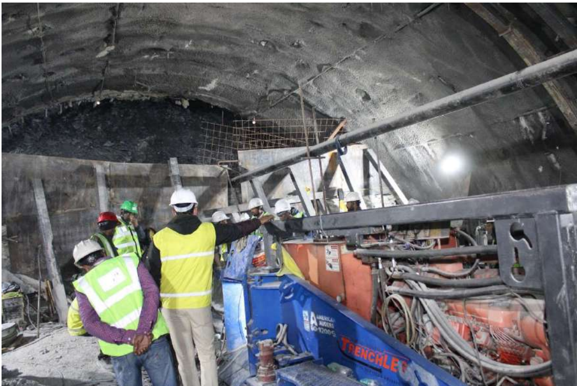
Figure 8 shows the Horizontal Auger Machine arriving at the tunnel site and strategizing for establishment.
