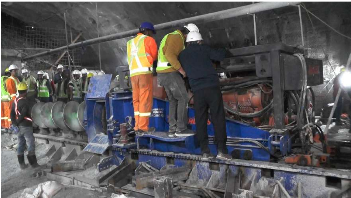
Figure 12 captures the commencement of the Augur Machine's operation, signalling the initiation of its functional activity.
