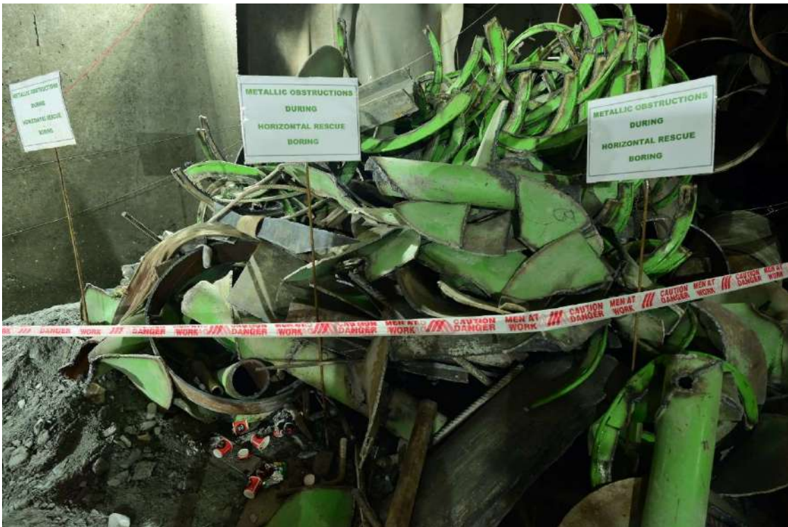
Figure 20, The occurrence of a metallic obstruction is depicted during the process of horizontal drilling. This visual illustrates a hindrance in the drilling operation caused by a metallic object, highlighting the challenges and considerations involved in the drilling process.
