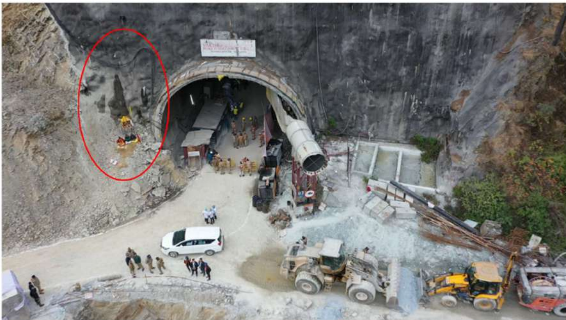
In Figure 18 , the site is portrayed with a red-coloured circle highlighting a subtle water seepage from the ground. This minor concern was addressed promptly at that specific moment.
