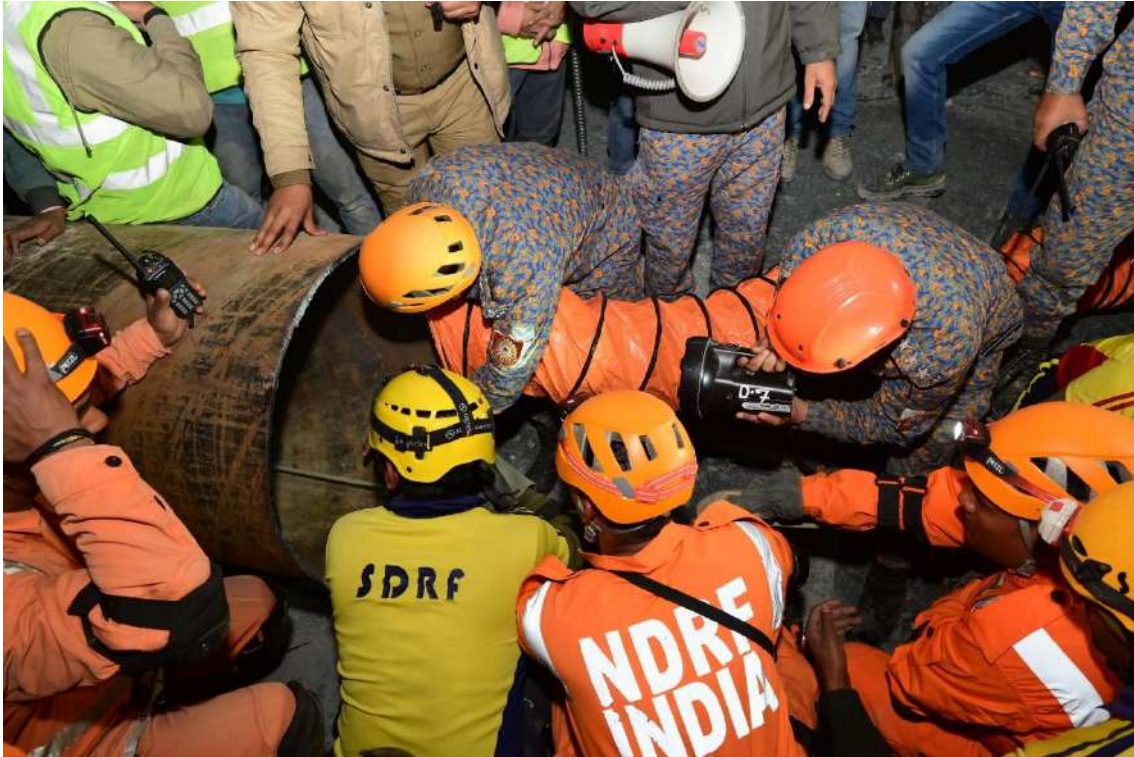
Figure 27 displays an individual arriving from inside the collapsed Silkyara Tunnel.
