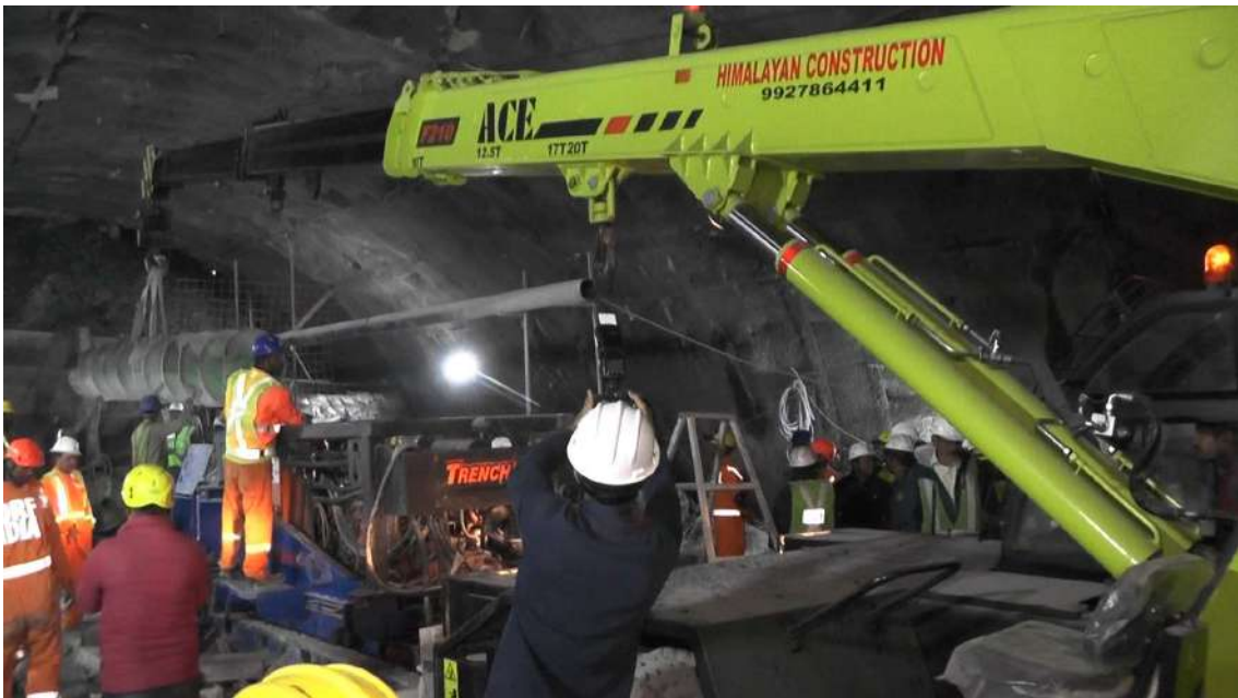
In Figure 10, dated December 14, 2023, the Auger Machine Blade has been positioned to facilitate horizontal drillings, marking a significant step in the operational process.
