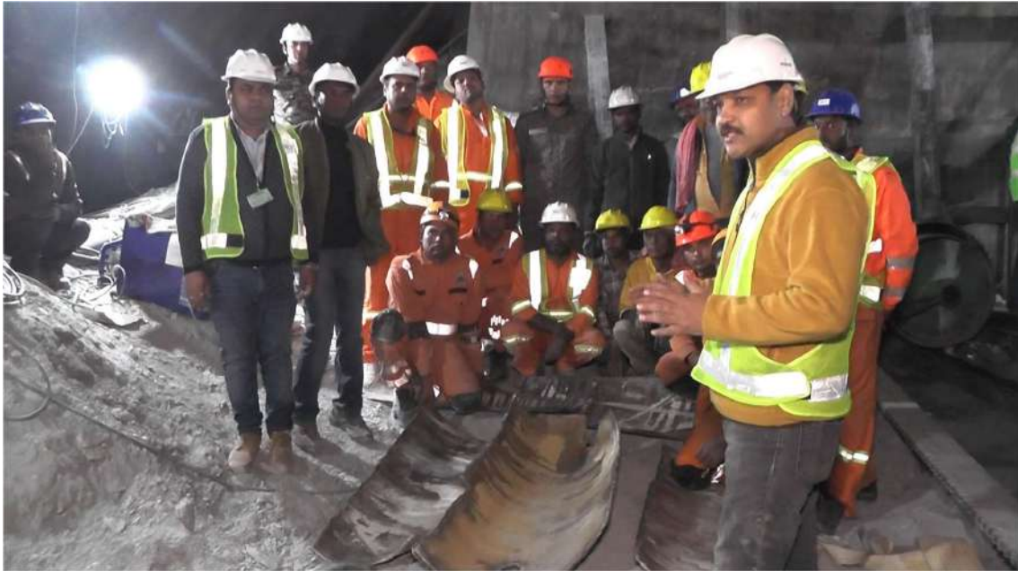
Figure 9 Planning is underway for the removal of debris, and the procedure is being explained.
